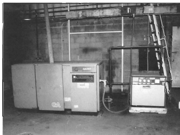
50 H.P. Rotary Compressor
