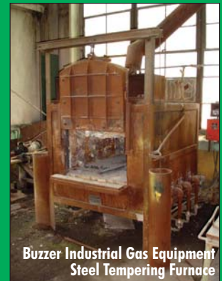
Buffalo Steel Forging Furnace
